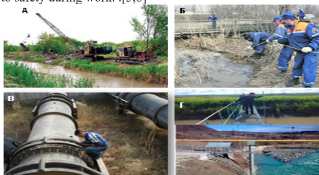
Figure 1. Working processes performed at the objects of the hydro-reclamation system.
