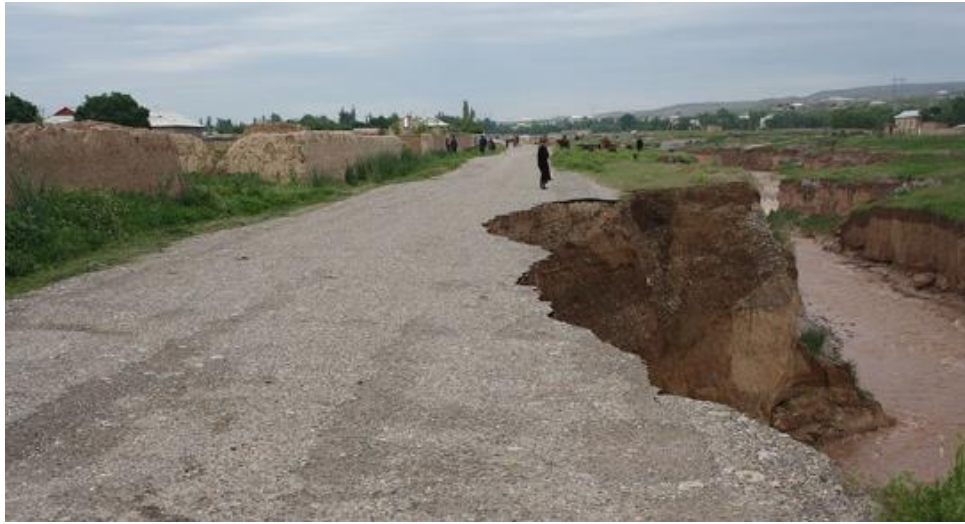
Fig. 1. Collapse caused by natural causes.
